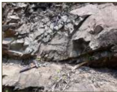
Figure 8. Highly jointed diorite. (Loc. N 25° 22' 28"; E 97° 44' 10.1")
